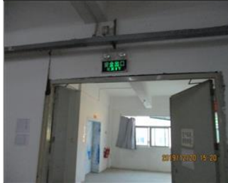
Photo of fire safety equipment Emergency exit sign and emergency light.JPG
