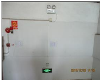
Photo of fire safety equipment Evacuation indicator sign.JPG
